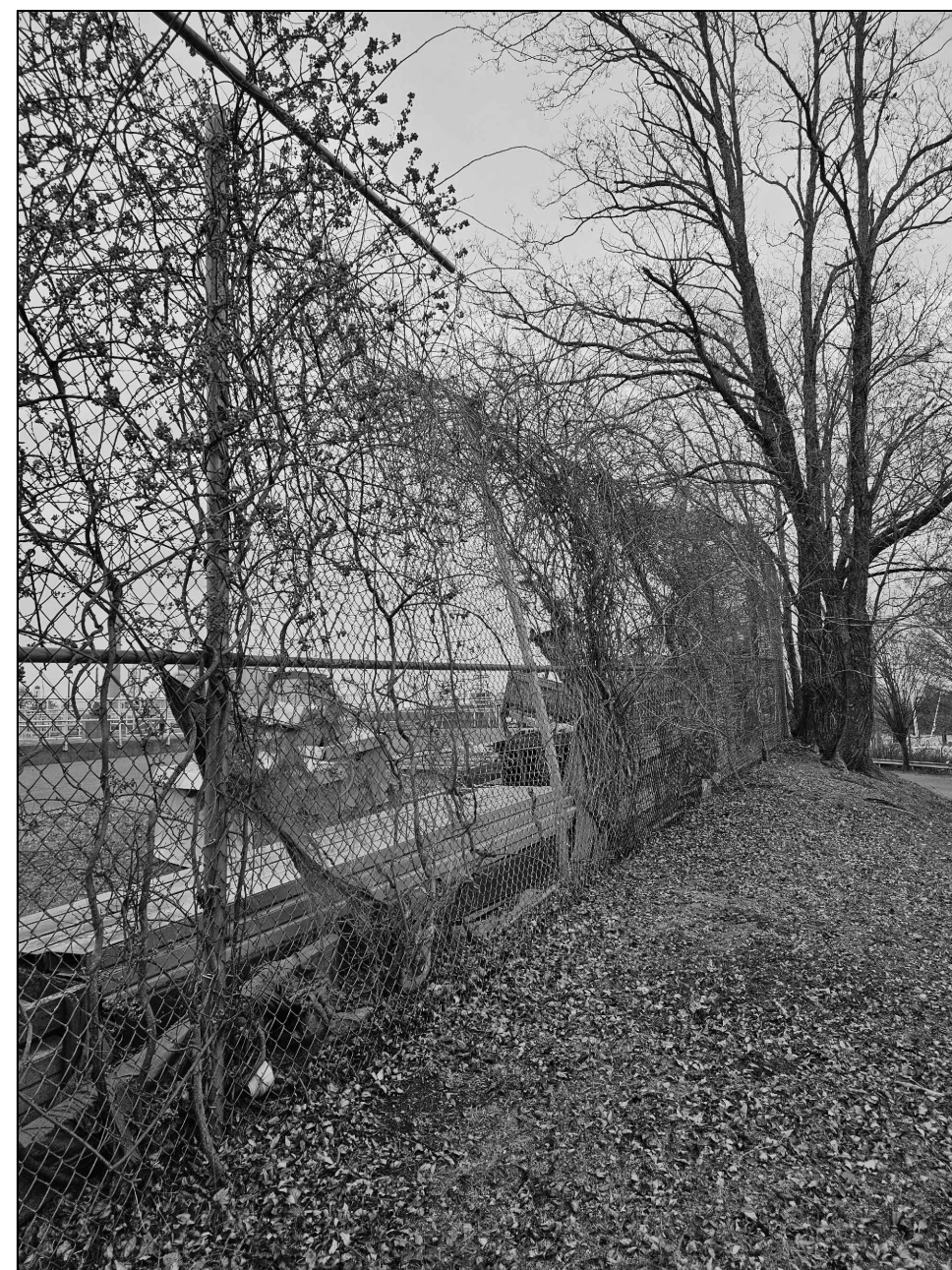
IMAGE 3: REPLACE FENCE POSTS, FABRIC, AND RAILS TO RESTORE FENCE INTEGRITY: APPROX. 30 LF
