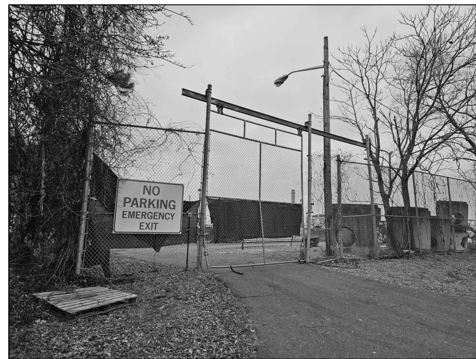
IMAGE 2: REPLACE TIES AT BOTTOM OF SLIDING GATE
