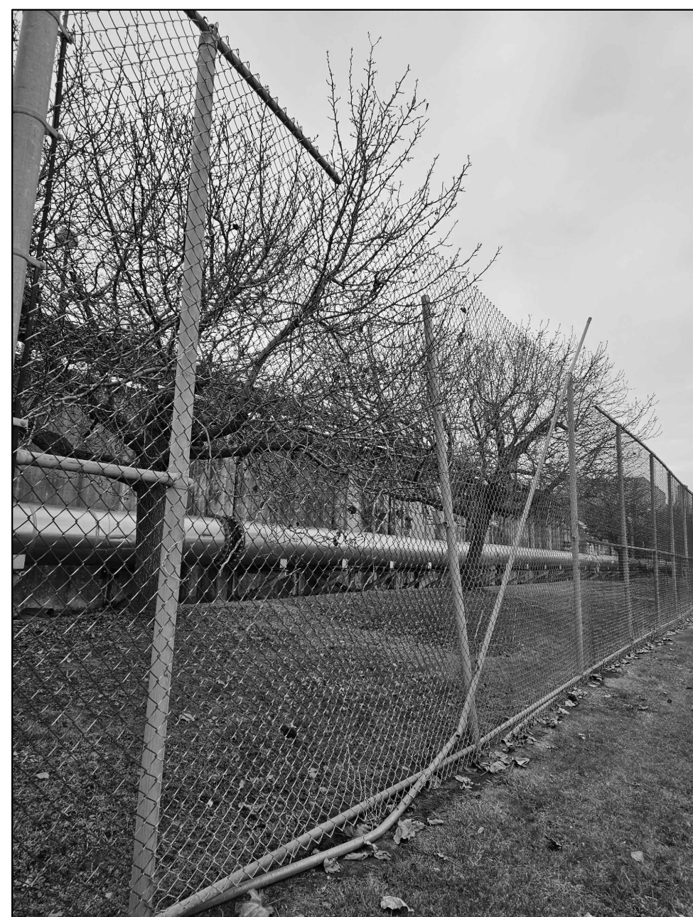
IMAGE 5: REPLACE FENCE POSTS, FABRIC, AND RAILS TO RESTORE FENCE INTEGRITY: APPROX. 25 LF
