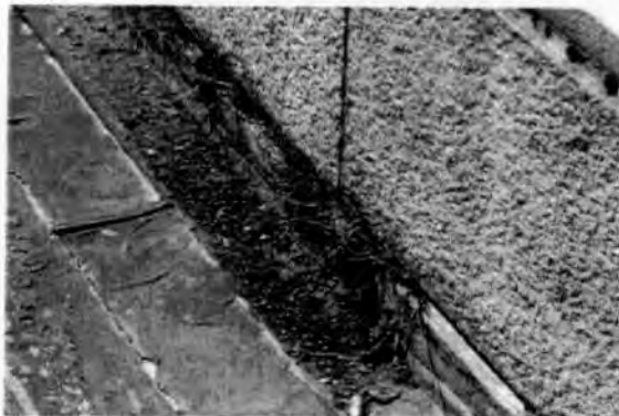
Photo 6: Deteriorated Copper Gutter w/ Grass
