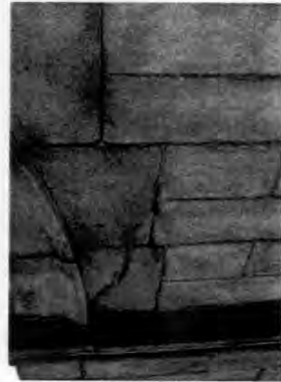
Photo 9: Step Crack at Arch Base
