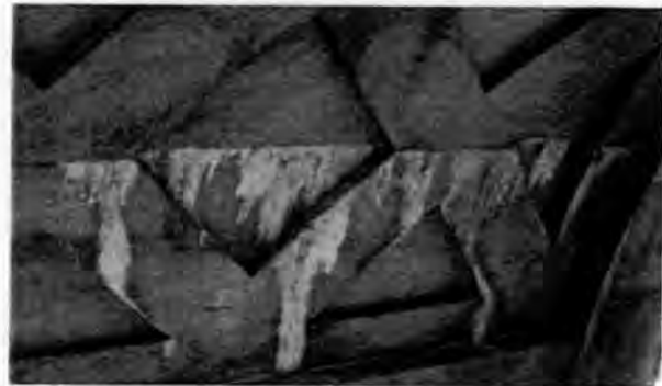
Photo 10: Calcium Deposits on Ceiling Panel
