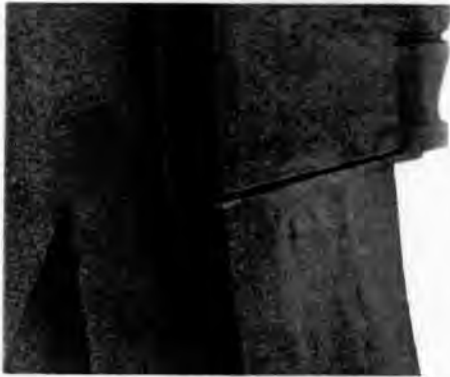
Photo 8: Missing Mortar at Keystone
