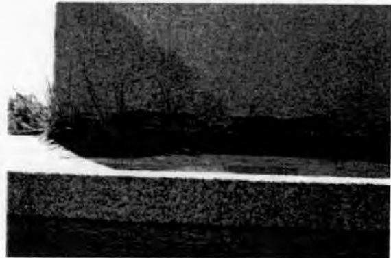
Photo 7: Missing mortar between Stones
