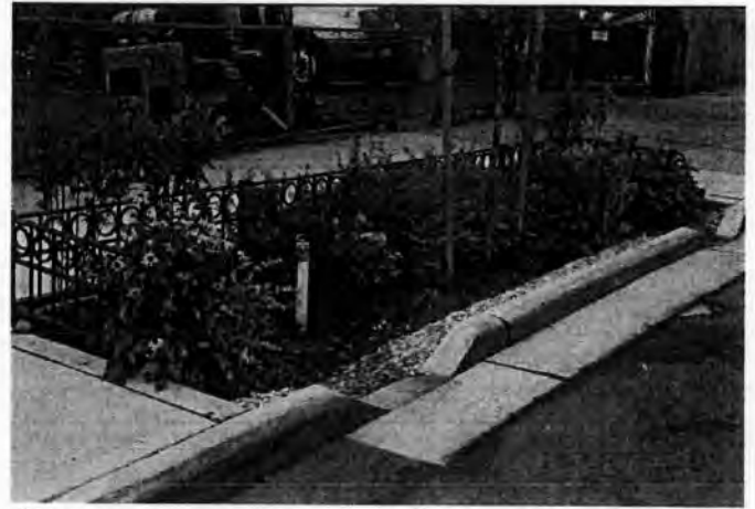
2) Here is shown the curb profile that lets gutter water detour into a planter where it can infiltrate or deposit pollutants and suspended solids (clay, sand, gravel, etc.).
