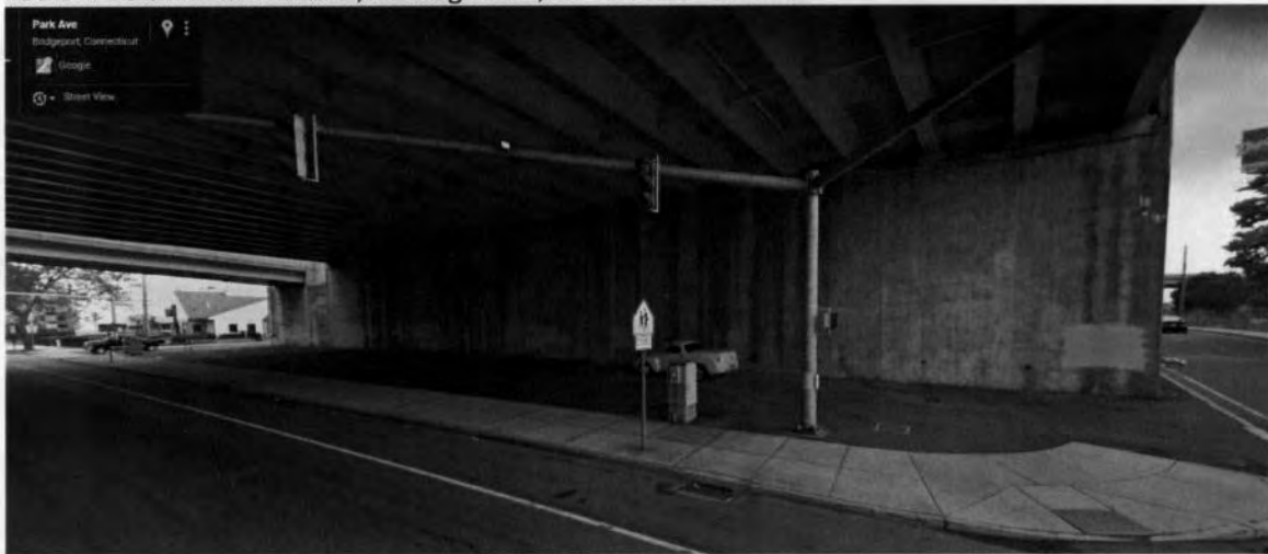
#95-B: I-95 and Park Avenue, looking north, east side of Park Ave
